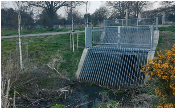
Two-stage 'self-cleaning' grille several times larger than the pipe itself – designed for large flood storage areas with high flows
